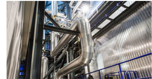
Technical insulation solution used in Vantaa Energia waste power plant.
